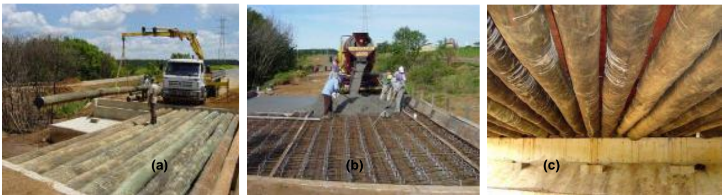
Fig. 2. Composite slab deck (Campus II USP Bridge, Brazil – 12 m span): (a) craning of log beams into position; (b) concrete placement; (c) bottom view
