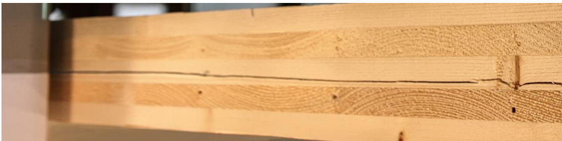
Fig. 10. Failure due to longitudinal shear occurred as shear stress parallel to the grain
