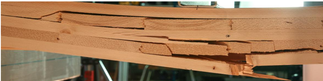
Fig. 8. Bending failure due to tension in the lowest outer layer
