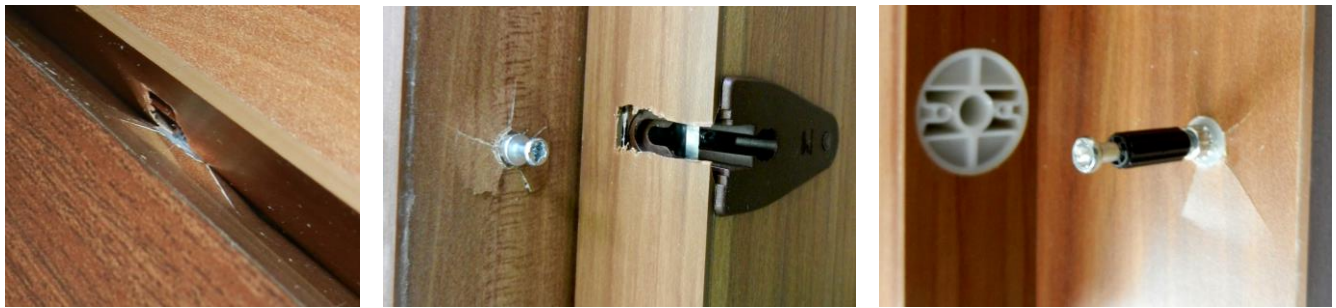
Fig. 5. a) Deformation of joint type D in compression; b) Deformation of joint type A in tension/compression; c) Deformation of joint type E in tension/compression
