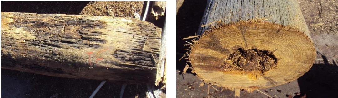
Fig. 2. Rot in the previously buried length
