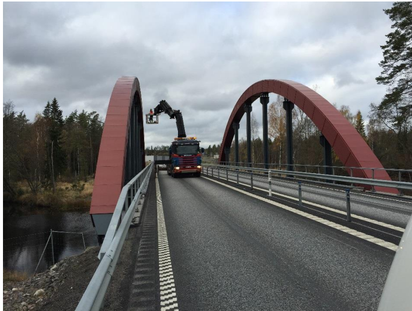
Fig. 7. Mounting a sensor on the south arch from the aerial work platform
