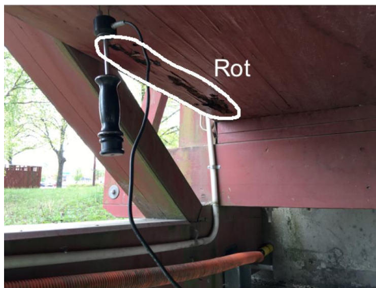
Fig. 2. The bottom of a pedestrian bridge with severe decay shown in the outer beam
