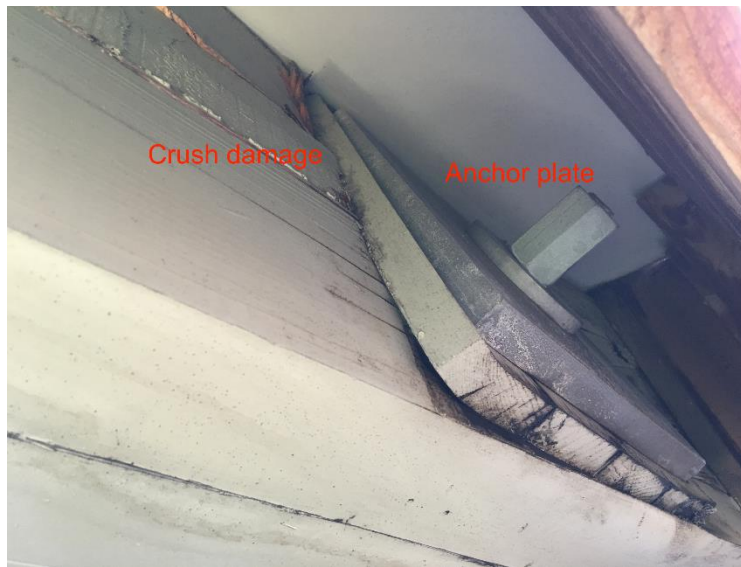
Fig. 1. Anchor plate crushing a rotten glulam beam
