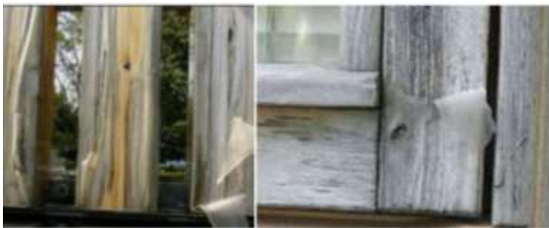
Fig. 3. Delamination of clear coating on wood (Evans et al. 2015b)
