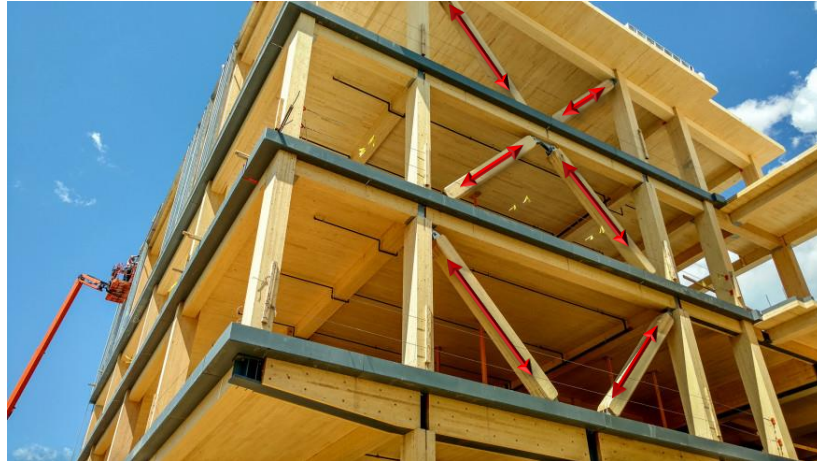
Fig. 2. A combined glulam and CLT structure. Glulam beams oriented at \pm 45^\circ provide structural wind load resistance (Photo used with permission from Alexander Schreyer/UMass)
