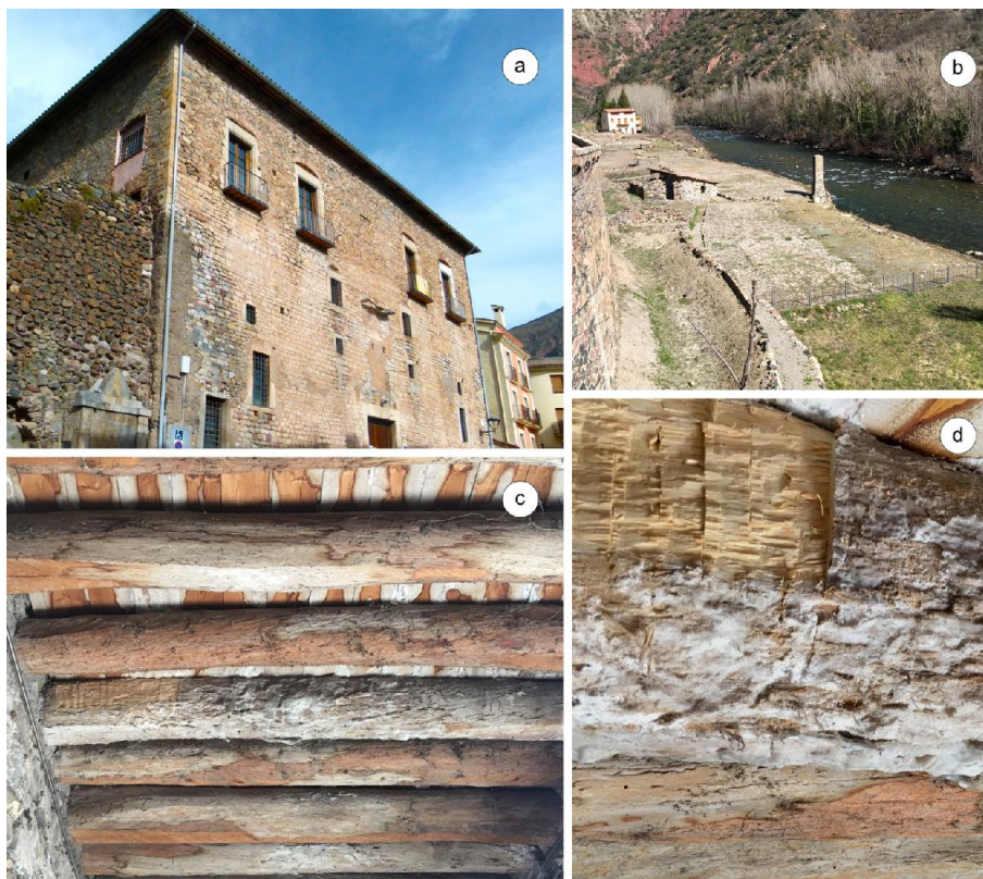
Fig. 1. a) Real Alfolí salt storehouse – Gerri de la Sal, Lleida (Spain); b) remains of the former saltworks on the banks of the Noguera Pallaresa river; c) wooden framework beam in contact with salt for 300 years; and d) sample extraction site, surrounded by accumulated salt
