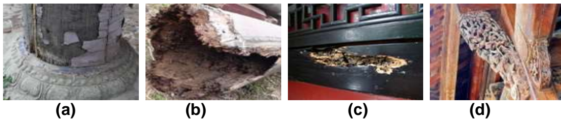
Fig. 1. Damaged characteristics of (a) decay, (b) hollow, (c) insect attacks, (d) crack
