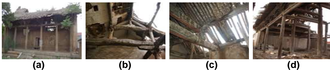
Fig. 2. Destruction of wooden structures in (a) Dongyue Temple, (b) Jade Emperor Temple, (c) Puming Temple, (d) Xia Jin Confucian Temple
