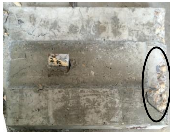
(c) Spalling of concrete
