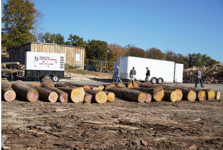
Fig. 2. The electric generator and portable steam/vacuum treating system at Polo Pallet/Mill Creek Lumber, Elkton, Maryland
