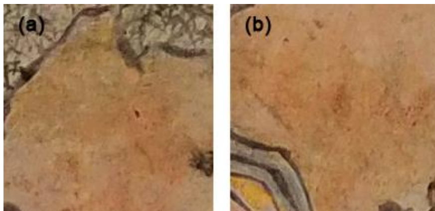
Fig. 5. The pigments layer of the Kaiping Diaolou pigments (a) Unrestored, (b) Restored
