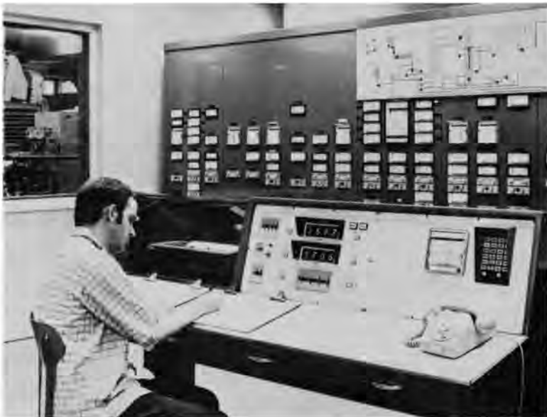
Fig. 7 —Process operator console developed at Billerud
