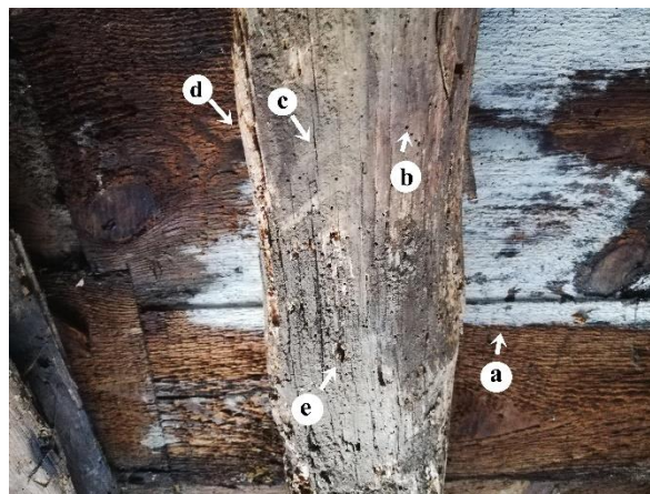
Fig. 5. Joist; a – Fungal attack, b – Bore holes of insects, c – Cracks in wood surfaces, d – Softened and bleached color, e – Large voids
