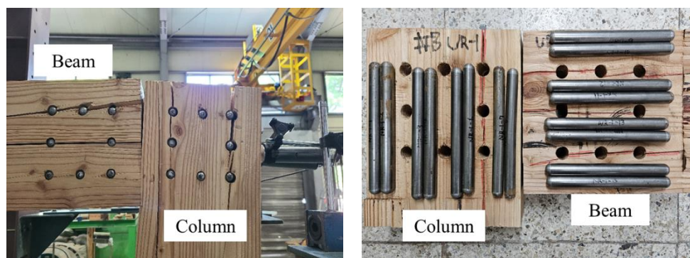
Fig. 10. Failure modes of laminated timber frame UR
