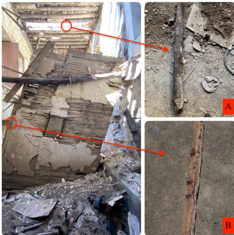
Fig. 2. The locations from which the wooden samples were extracted are as follows: A) The first sample was taken from the wooden ceiling of the ground floor; B) The second wooden sample was taken from the timber frame
